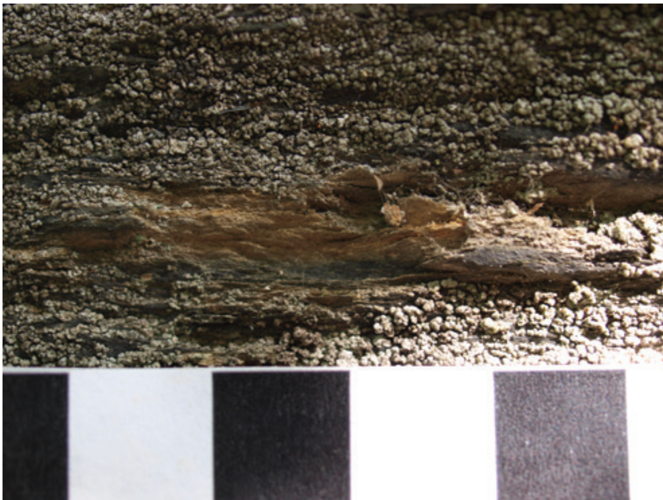
Figure 13: Typical destruction in the picture area. Such damages can be observed since 2014 (photo: W. Welker).
